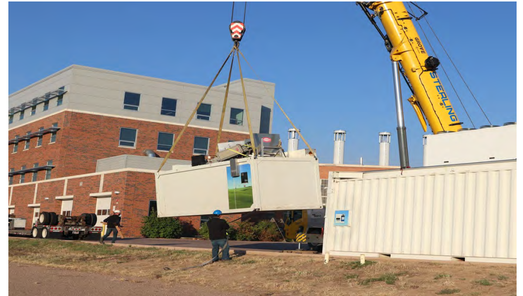
New hydrogen production facility at the Powerhouse Energy Campus
